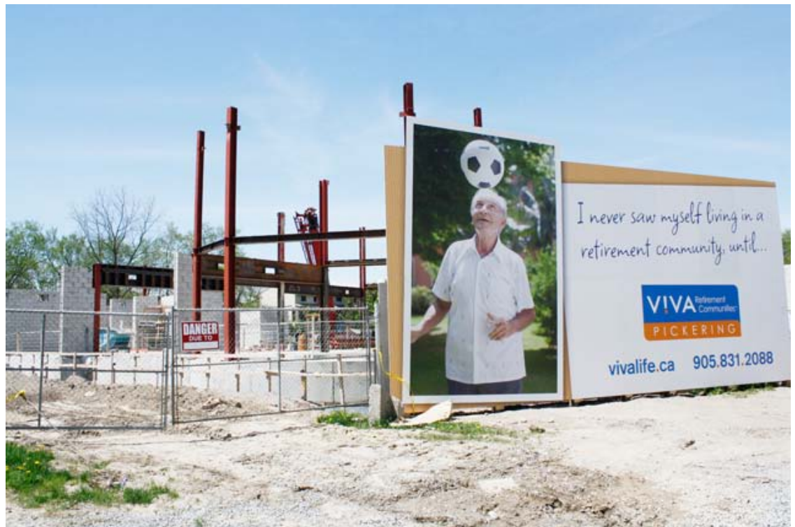
(Above) Steel and concrete block rise above hoarding at new VIVA facility
